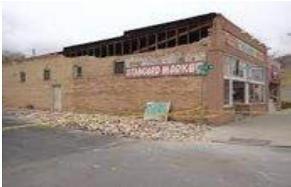
Eartquake Damage from Unreinforced Masonry
